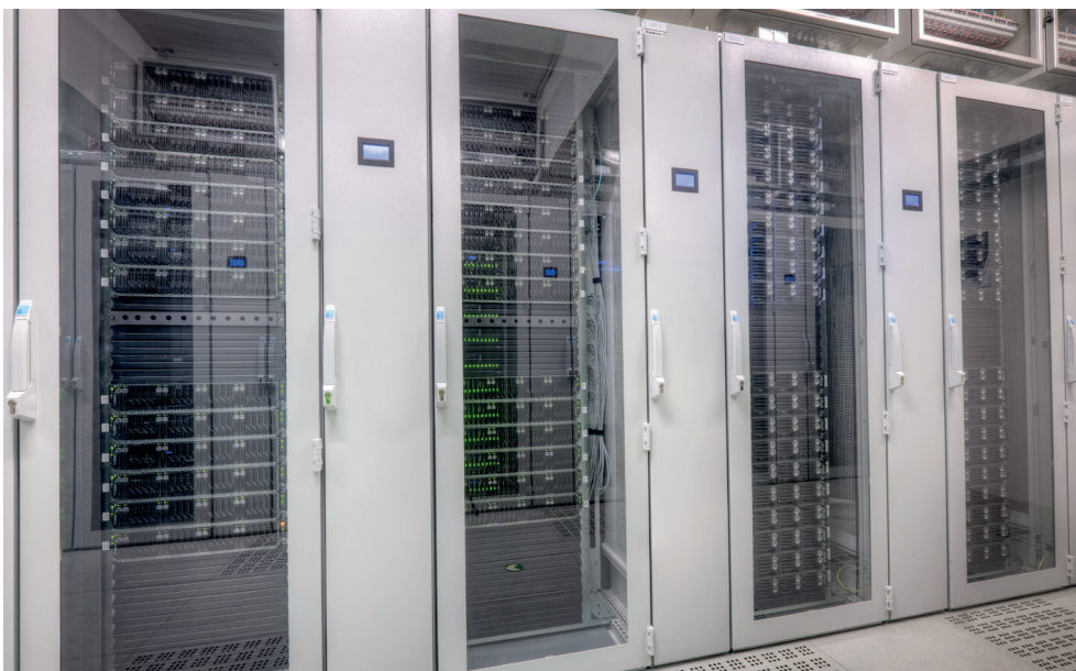
Four water-cooled racks containing servers.
