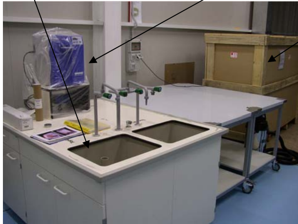
Washstand with high-purity water supply
