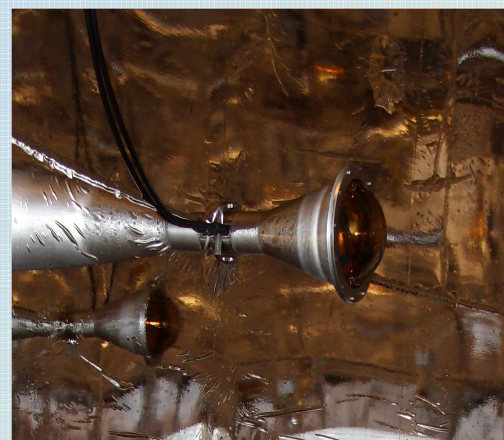
Mounted capsule on the wall of the water tank
