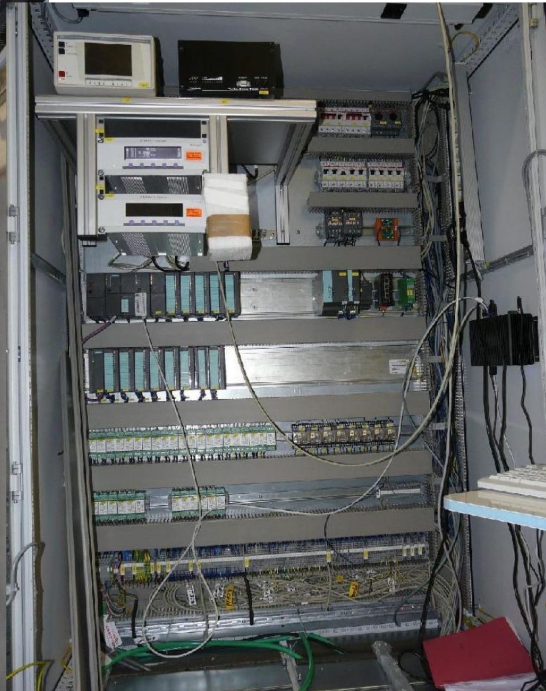
PLC cabinet connection to LNGs safety ready
